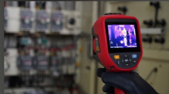
Power Distribution Cabinet Inspection
