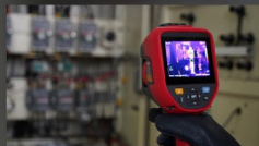
Power Distribution Cabinet Inspection
